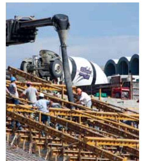
Take a “peek behind the fence” to see progress on the new Richard L. Jantz Stadium at www.sckans.edu/stadium .
